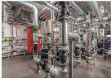
Municipal heating system
