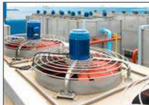
Fans and water pumps
