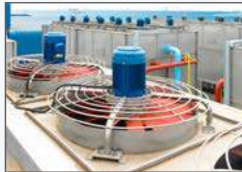
Fans and water pumps
