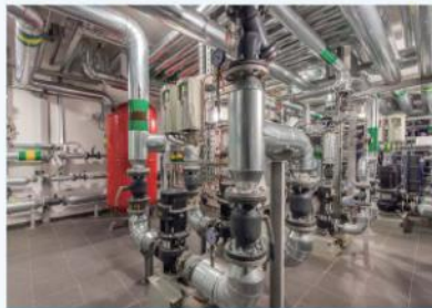
Municipal heating system
